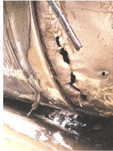
Exhibit 2: failed gasketed joint
